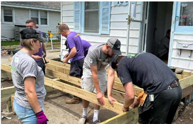
F&G team members collaborate to build a deck in partnership with Rebuilding Together
